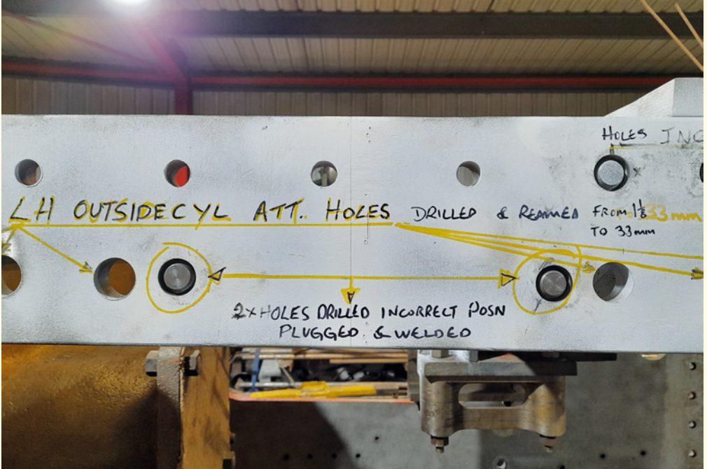
Example of mapping the frame repairs. This is kept on record for future reference.
