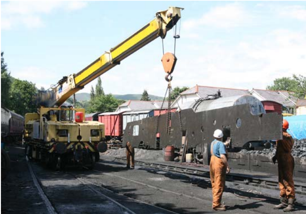
The Llangollen Railway's diesel crane was used for all the lifting and handling of the frame plates.
